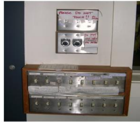
Turn on church ceiling fans Turn on lights in church
