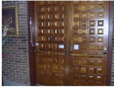
Front Entrance Door
