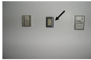
Clrm #18/19 Bldg Thermostat
