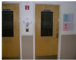
Clrm #18/19 Bldg Thermostat
